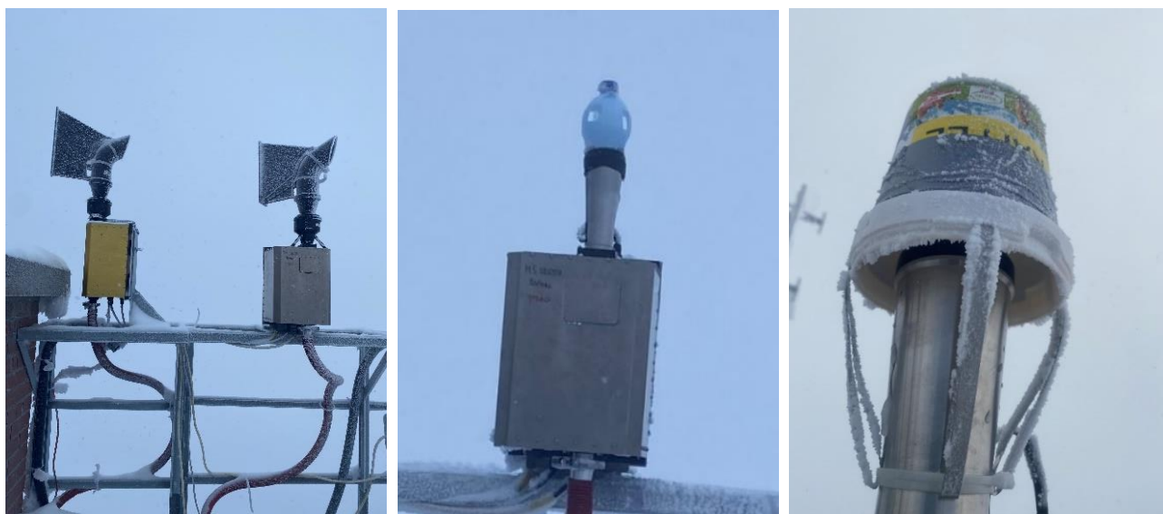
Figure S1. FM_CAS installation during the ECCINT-INT01 campaign, showing (left) swivel inlet, (middle) PET bottle inlet with four openings, and (right) bucket-type inlet.
