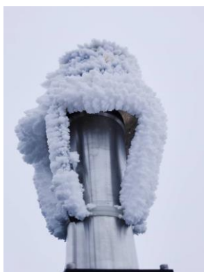
Figure S2. Bucket-type inlet during operation with significant riming. Despite ice accumulation, airflow remained sufficient to allow continuous sampling.
