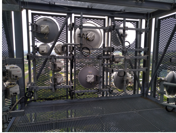
Figure 4. Example of a real rooftop CML installation. The units experience different solar exposure and shading conditions despite being located at the same site.
