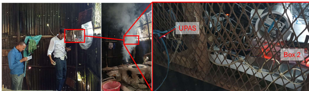
Figure A4: Sensor and gravimetric instrument installations at location Kitchen 1.
