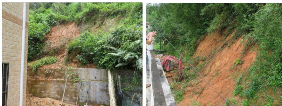
83 84 Figure 2: Photos of the on-site investigation of shallow landslides.
