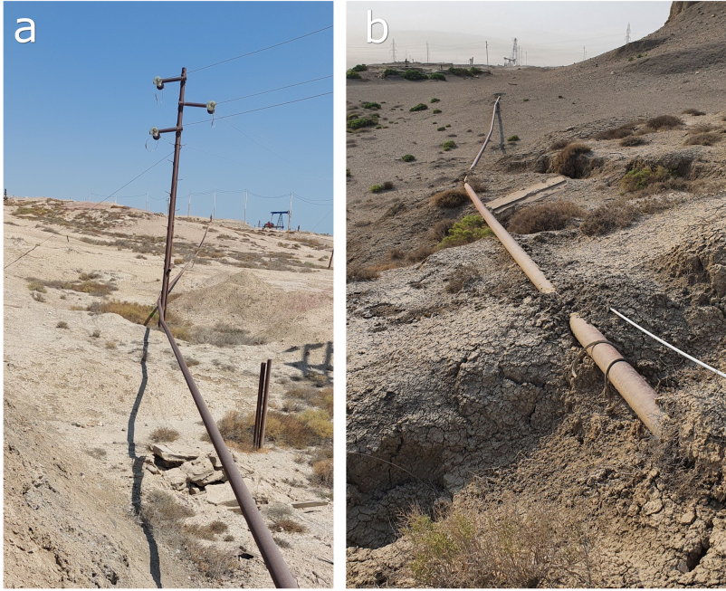
235 Figure 5: Example of infrastructures built across the creeping mud flow at Lokbatan MV. (a-b) ongoing flow movement 240 causes deformation of the pipeline.
