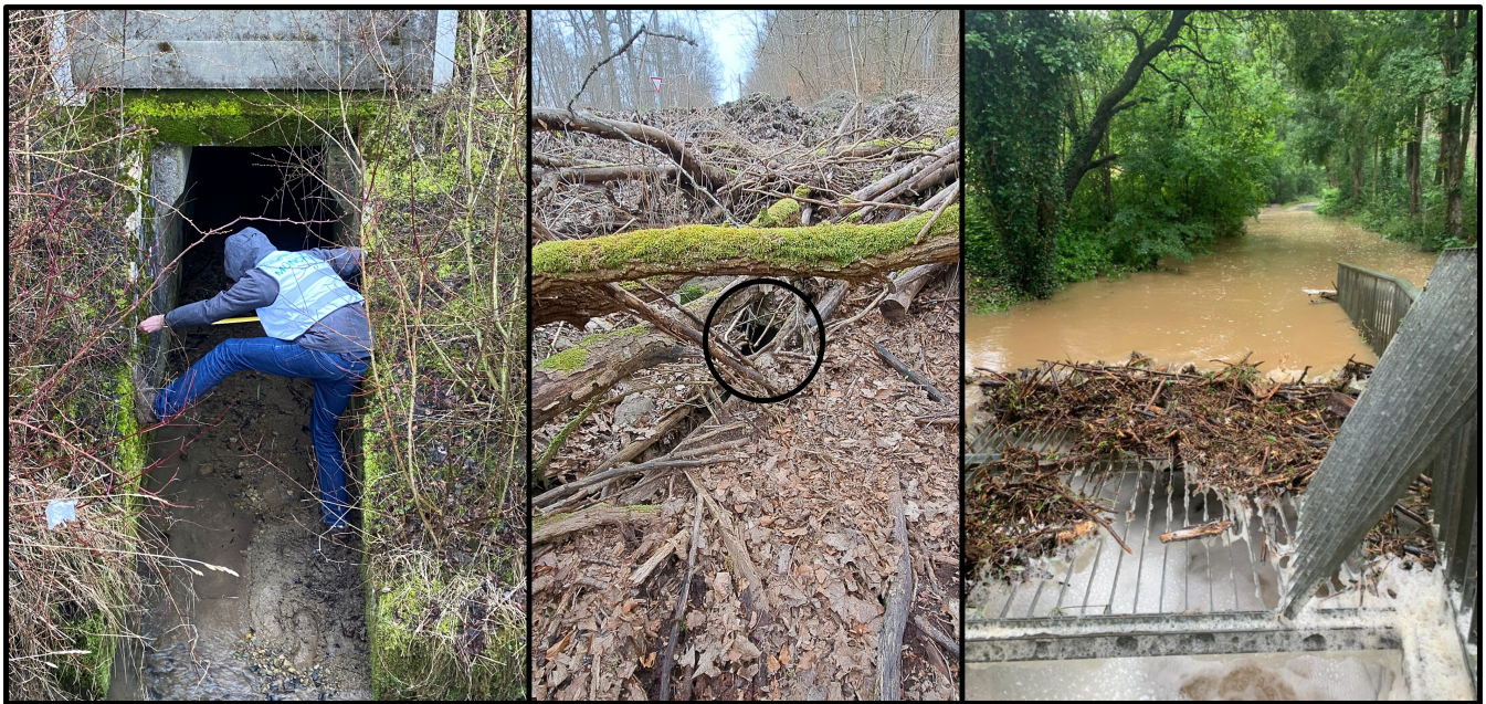
Figure 4. left: inspection of an unsurveyed culvert with slight sedimentation, middle: extreme logjam in front of an unsurveyed culvert (see black circle for culvert location), right: blocked culvert during the flood event at 9th of July, 2021 (Feuerwehr Reichenberg (2021b), https://ff-reichenberg.de/einsatzberichte/1752-hochwasser-strasse-ueberflutet/ )
