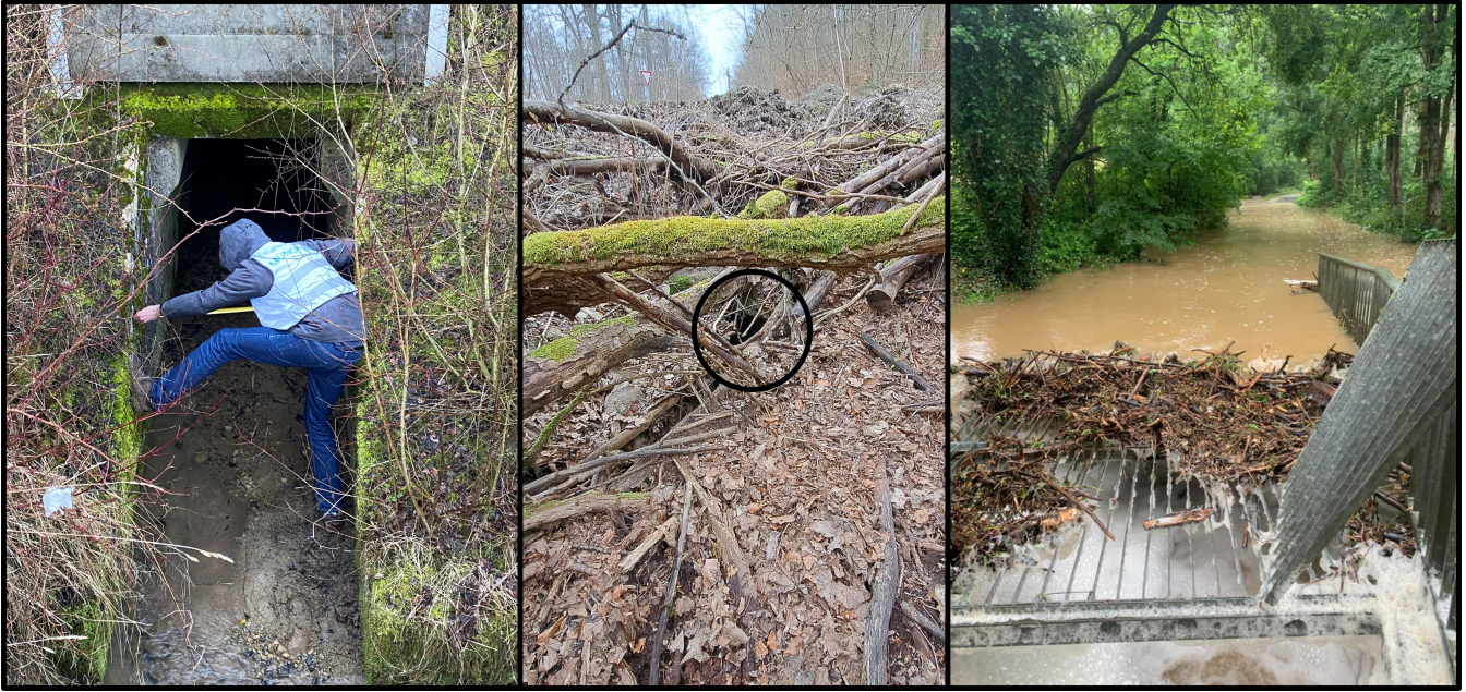
Figure 4. left: inspection of an unsurveyed culvert with slight sedimentation, middle: extreme logjam in front of an unsurveyed culvert (see black circle for culvert location), right: blocked culvert during the flood event at 9th of July, 2021 (Feuerwehr Reichenberg (2021b), https://ff-reichenberg.de/einsatzberichte/1752-hochwasser-strasse-ueberflutet/ )
