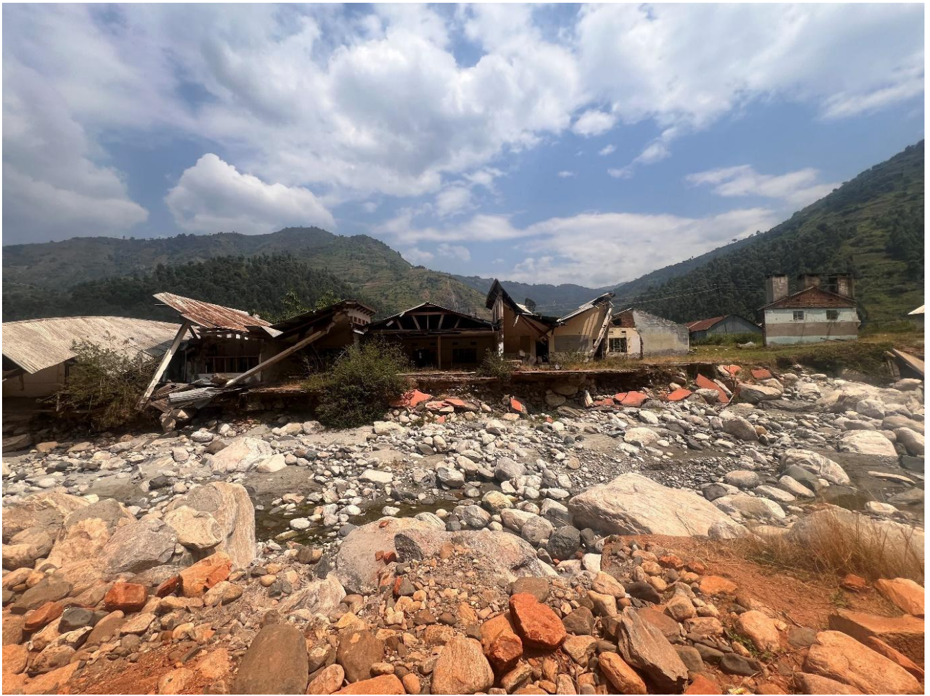
Figure F2: Riverbank style erosion of house foundations in Kilembe, 0.20603N, 30.00822E – 24 July 2024.
