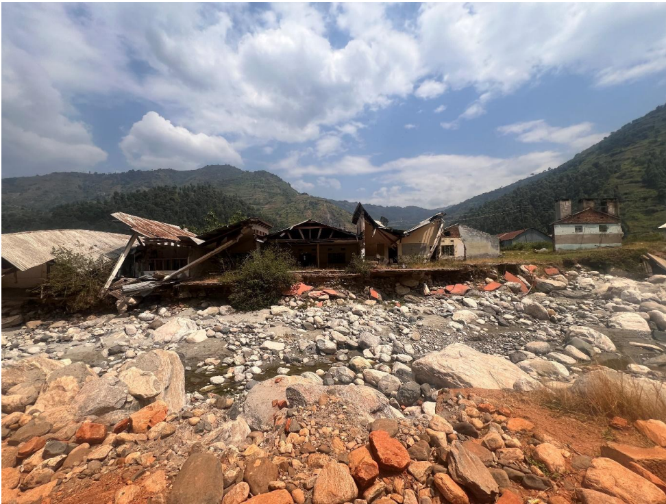
889 890 Figure F2: Riverbank style erosion of house foundations in Kilembe, 0.20603N, 30.00822E – 24 July 2024.
