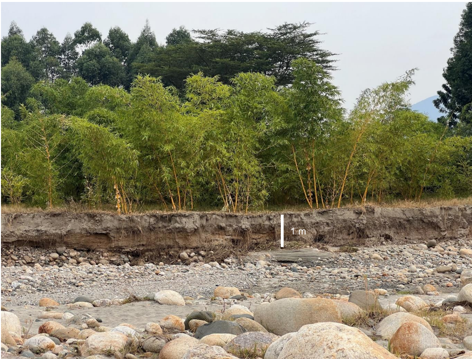
914 915 Figure H1: 0.18981N, 30.07408E, 26 July 2024 (damaged bamboo nature-based solution).
