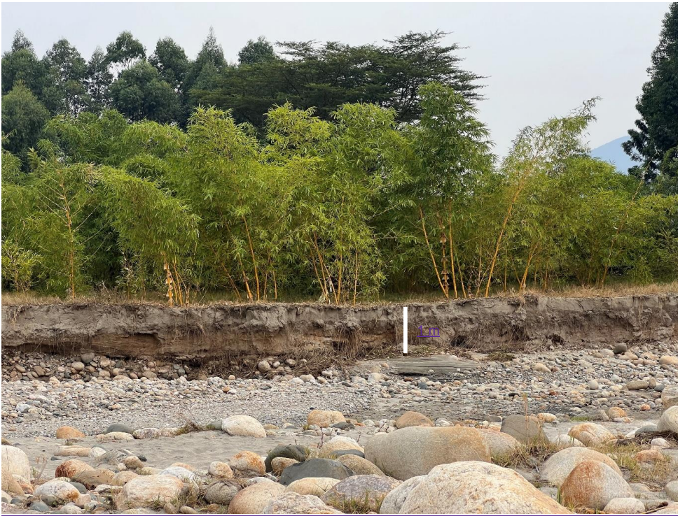
Figure H1: 0.18981N, 30.07408E, 26 July 2024 (damaged bamboo nature-based solution).
