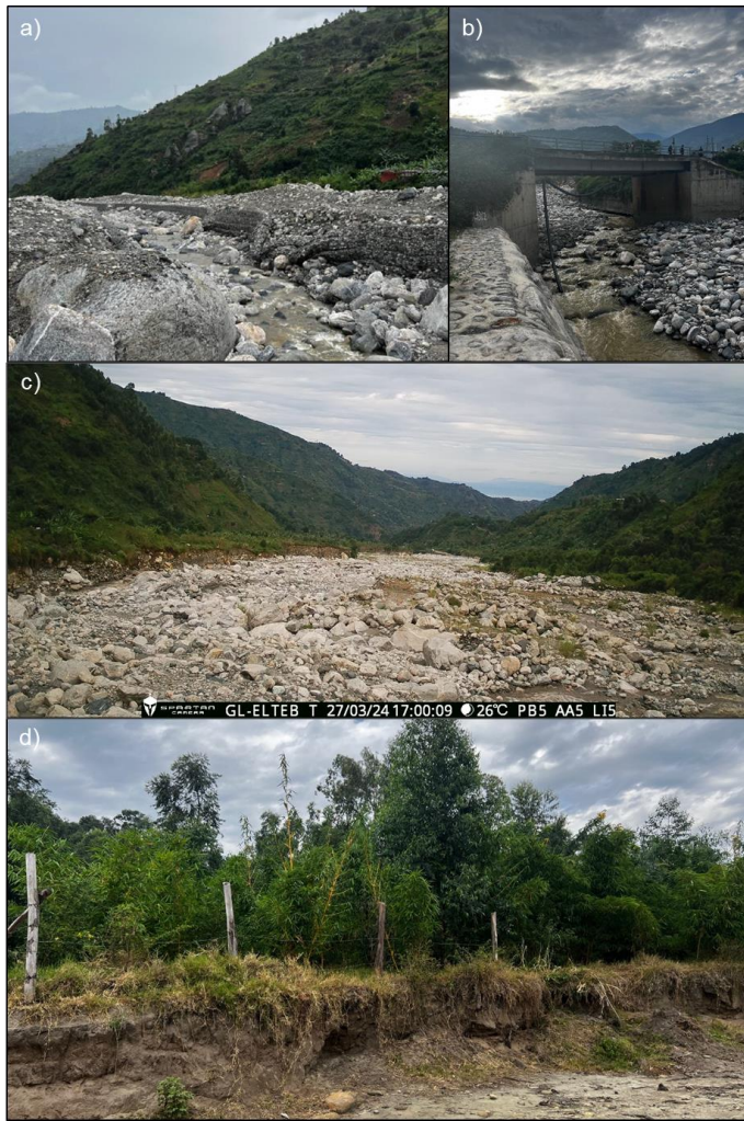
Figure L4MI – Photographs taken during June 2023 field reconnaissance: a) collapsed gabions adjacent to Kilembe town (for scale: 8 m channel width); b) channelisation using concrete embankments in Kilembe town centre (10 m channel width under bridge); c)
