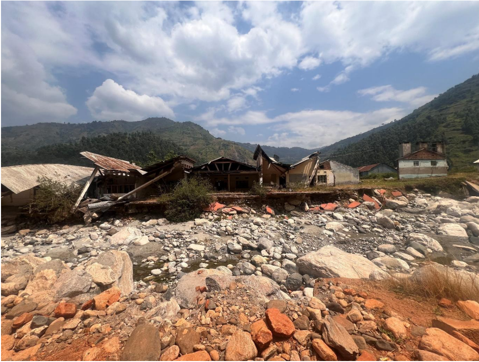
960 961 Figure F2: River cliff style erosion of house foundations in Kilembe, 0.20603N, 30.00822E – 24 July 2024. 962 963 964 965 966 967 968 969 970 971
