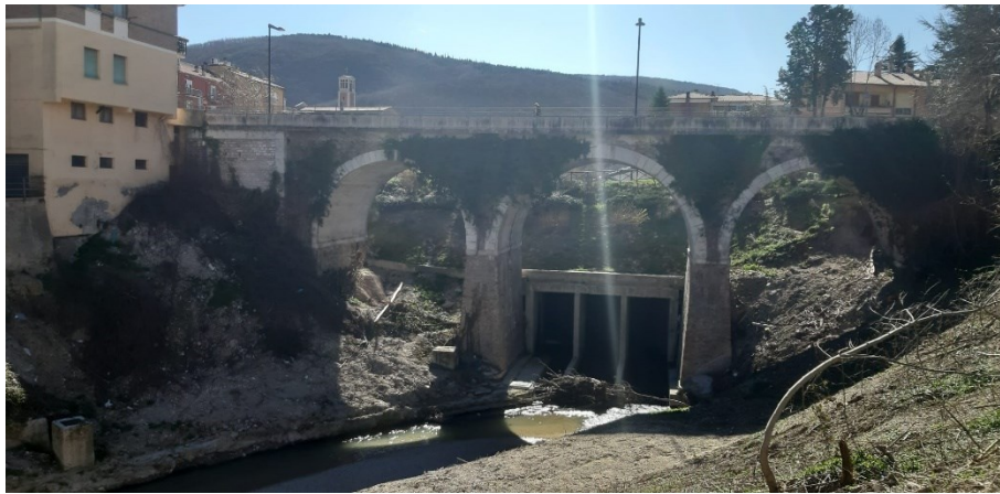
Figure 21: The Garibaldi Street Bridge saw from upstream with the evident, extreme reduction of the original flow section with a box-like structure (the markers on the wall on the left mark the hydrometric levels reached).
