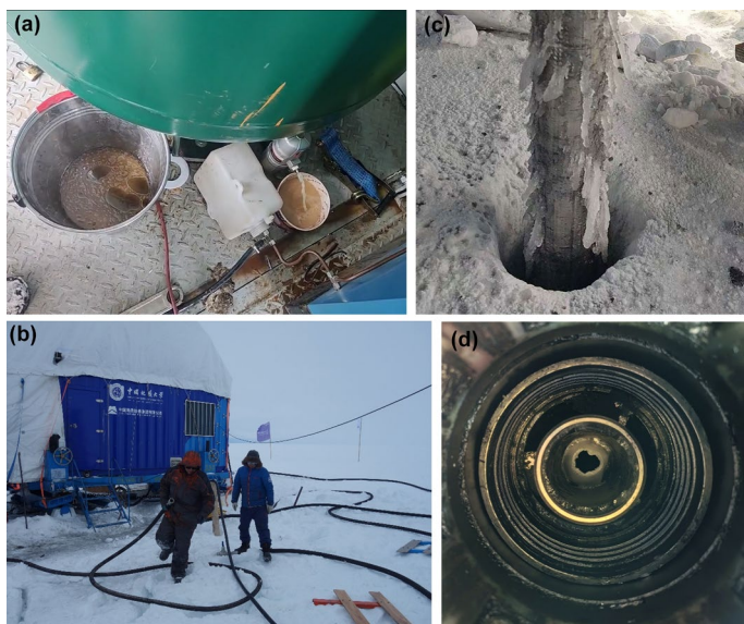
Figure 9: Test phenomena: (a) cyclone dust collector worked well in domestic test; (b) condensed water could not be discharged from the receiver; (c) burying the rubber hose into snow to cool compressed air; (d) condensed water refrozen on the outer surface drill pipe; (e) ice plug formed in drill pipe.
