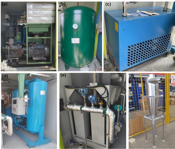
210 Figure 3: Main components of the air system: (a) air compressor; (b) air receiver; (c) freezing dryer; (d) desiccant 215 dryer; (e) air cooler, 1-flowmeter, 2-dew-point hygrometer, 3-manometer, 4-temperature sensor; and (f) cyclone dust collector.
