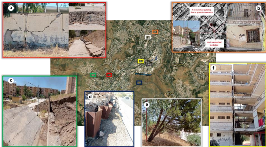
Figure 2 Field evidence of slope instability in the study area : a) Example of cracks in buildings and roads; b) Shallow landslide scarp in an urban setting, with an adjacent demolished structure; c) Failure of a concrete retaining wall; d) Sheet-pile retaining system exhibiting lateral bulging; e) Leaning tree signalling slope deformation; f) Example of inclined buildings
