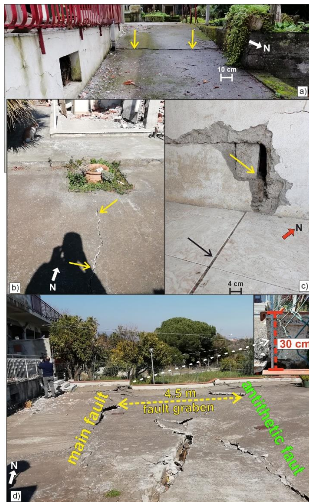
220 Figure 5: 26 December 2018 coseismic ruptures at Collegio Fiandaca trench site (see photos location in Fig. 4): a) ground rupture along a private road with few cm of offset; b) ground rupture which follows a damaged building wall, offset ~1 cm; c) 1.5 cm horizontal offset between two floor tiles continuing into the wall; d) fault graben on a private asphalt parking which extends over the wall and farmland.
