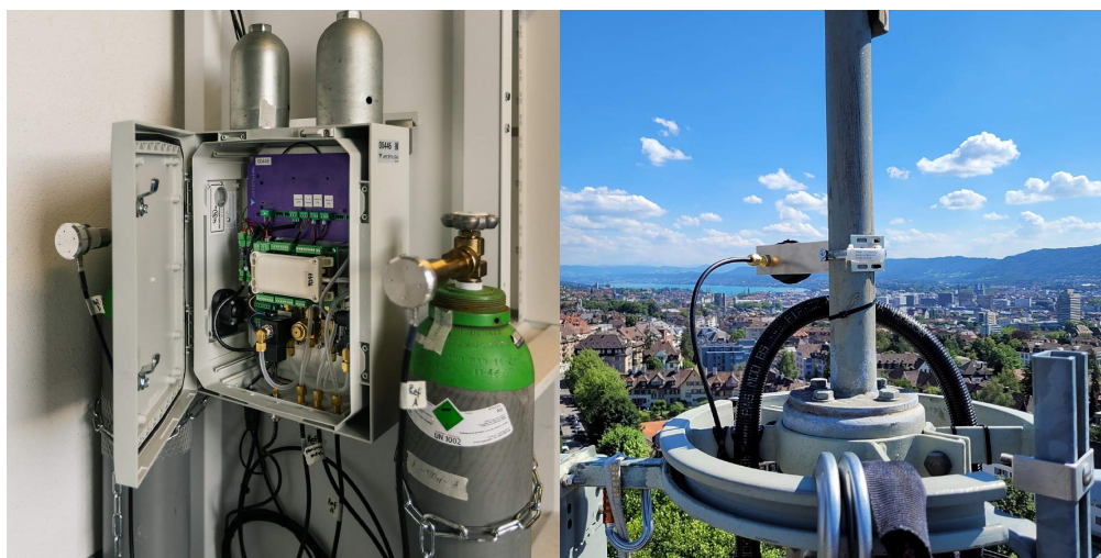
Figure A1. Examples of the CO 2 sensor's typical installations in the CARIN-ZH sensor network in Zürich city. The photograph on the left was taken by Pekka Pelkonen from ICOS RI.
