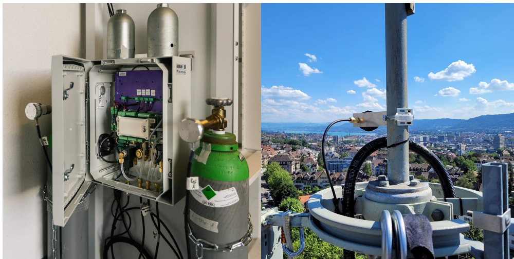
Figure A1. Examples of the CO 2 sensor's typical installations in the CARIN-ZH sensor network in Zürich city. The photograph on the left was taken by Pekka Pelkonen from ICOS RI.
