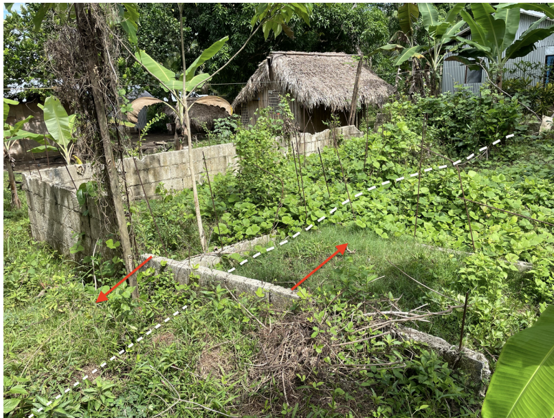
Figure S9: Pt FC4a. Unfinished house traversed by fault with deflected wall.
