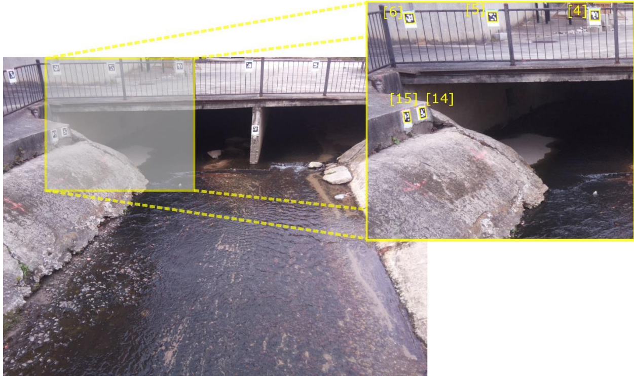
Figure 2 Visually illustrate where ArUco markers install and how they are detected.
