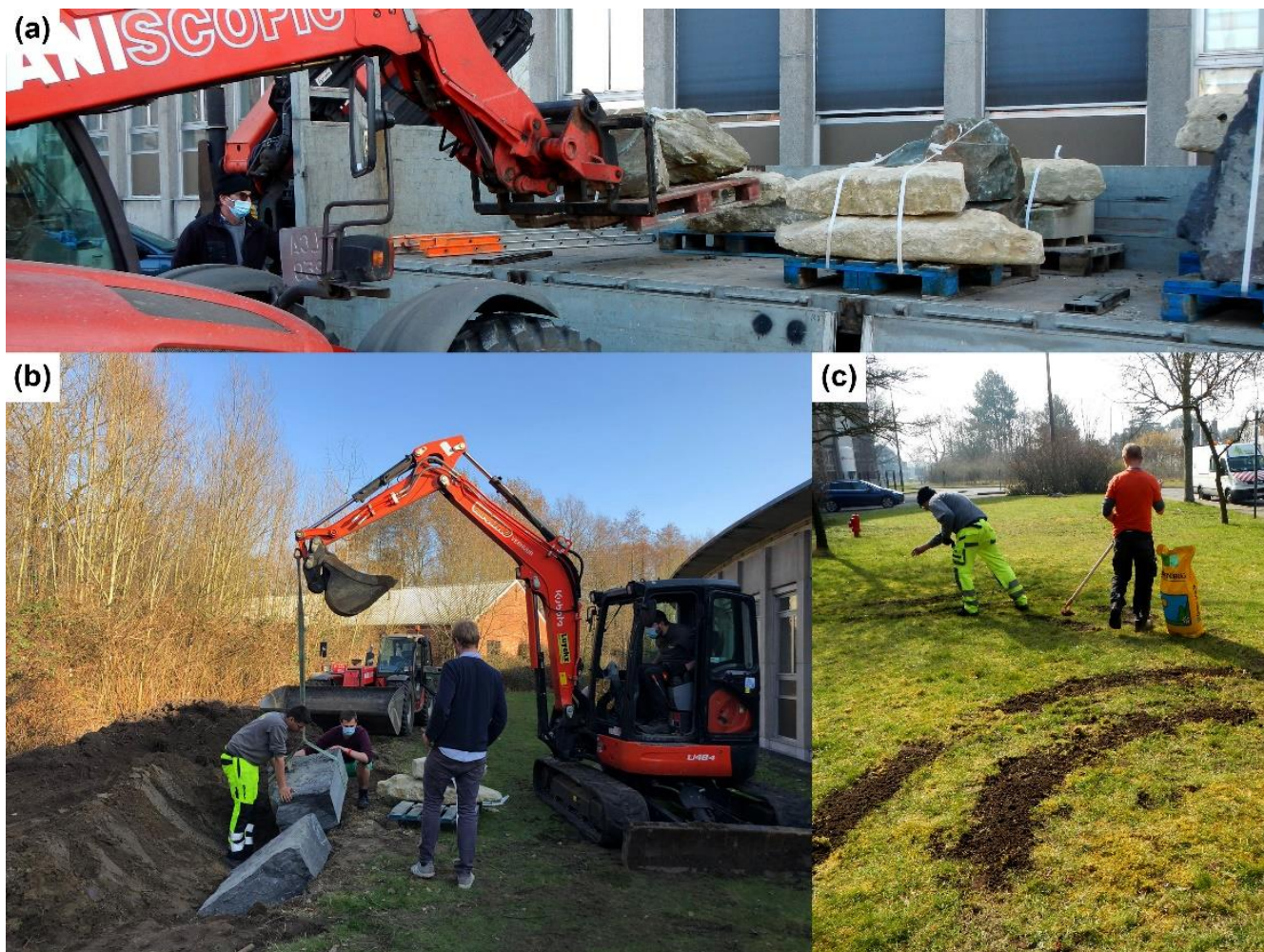
475 Figure 1 Installation of the Rock Garden at Ghent University. (a) Rocks were delivered in coordination with Monument NV and unloaded with the help of the Ghent University DGFB. (b) Rocks were installed, under careful supervision, using both human and machine power. (c) After installation, green areas were reseeded with grass or wildflower seeds to ensure full recovery of the green spaces.
