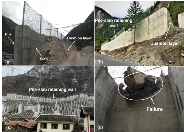
Fig. 1. PSRW in south-western China (a) Kongyu town (b) Jiuzhaigou nature reserve (c) Zhenjiangguan tunnel exit in Chengdu-lanzhou railway (d) Wenchuan-Maerkang expressway.
