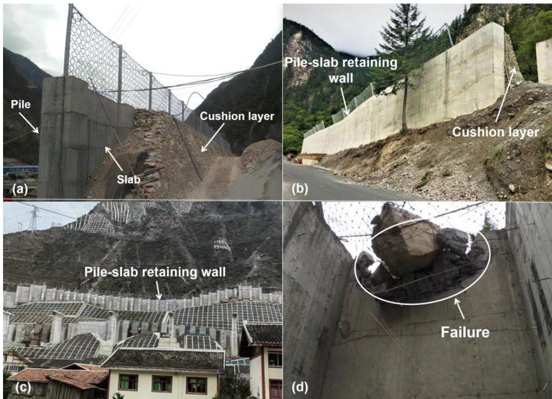
Fig. 1. PSRW in south-western China (a) Kongyu town (b) Jiuzhaigou nature reserve (c) Zhenjiangguan tunnel exit in Chengdu-lanzhou railway (d) Wenchuan-Maerkang expressway.
