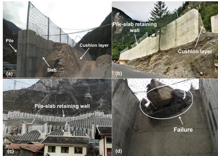
Fig. 1. PSRW in south-western China (a) Kongyu town (b) Jiuzhaigou nature reserve (c) Zhenjiangguan tunnel exit in Chengdu-lanzhou railway (d) Wenchuan-Maerkang expressway.
