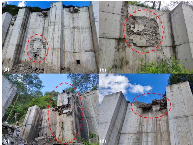
Fig. 2. Some PSRW in Zhangmu Town were damaged by falling rocks.
