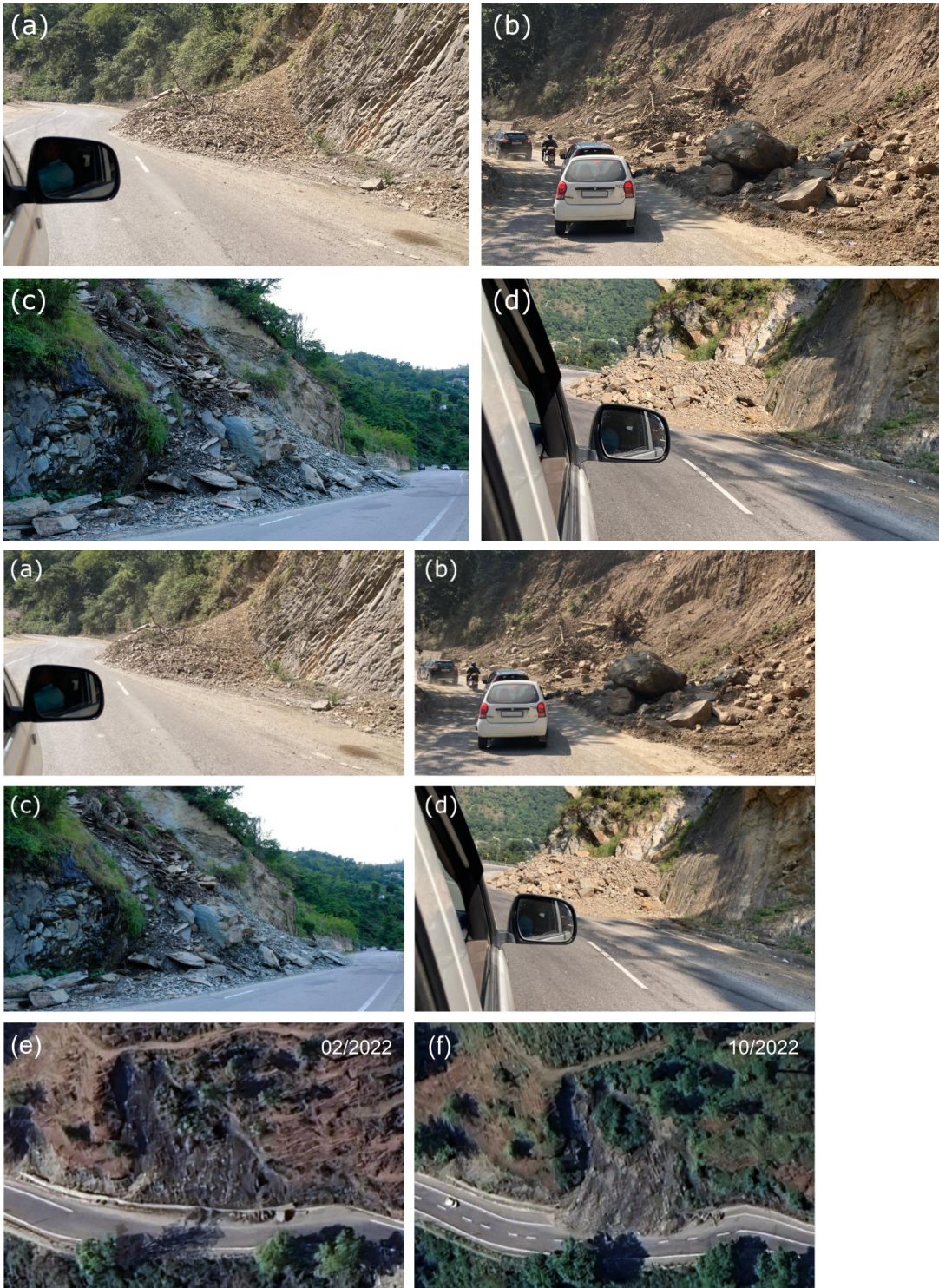
Figure 2: Examples of partially road-blocking landslides along the highway NH-7. Panels a) and c) show locations, where hillslopes parallel the foliation/bedding. Panels (e) and (f) show a landslide that was reactivated in the observation period.
