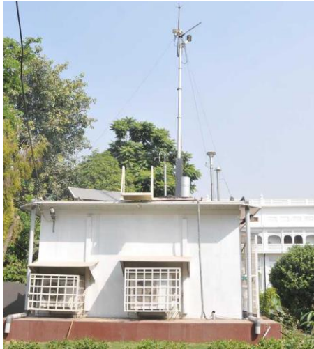
Figure 1: Meteorology monitoring station at Amritsar
