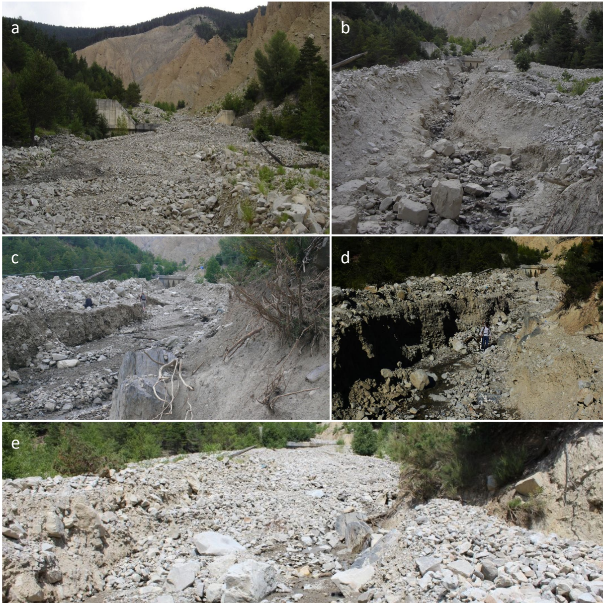
Figure 8. Pictures (from G. Piton) taken on the S_1 stations over 6 years a) channel filled in June 2009, b) channel deeply incised in July 2011, c) channel widened and partially refilled in June 2014 (person for scale), d) channel further incised October 2014 (person for scale), e) channel refilled in July 2014 (pictures from the authors)
