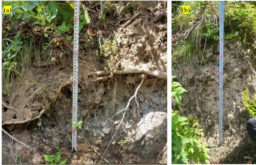
Landslide sidewall (north-facing slope). Near the middle and lower part of the landslide mass, the bedrock has been exposed.
