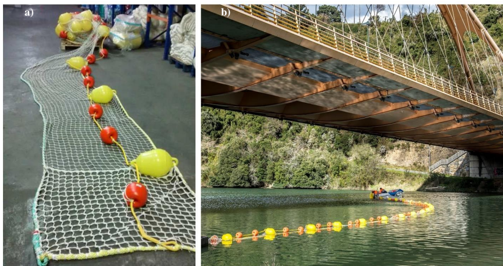
Appendix A. Floating barrier (a) and installation in Deba river (Gipuzkoa) (b)
